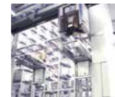
Automated Material Handling Systems for Clean Rooms -AMHS for Semiconductor Fab. -MCS (Material Control Systems)
